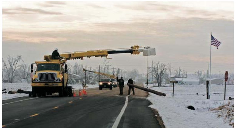
New-Mac linemen change out one of the more than 2,500 poles that were broken in the service area of Ozark Border Electric Cooperative.
