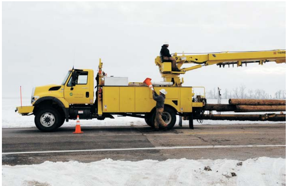
New-Mac Electric had linemen helping out Ozark Border Electric Cooperative, headquartered in Poplar Bluff, for nearly three weeks.
